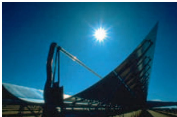
Power stations use trough shaped mirrors that concentrate the sunlight onto a pipe filled with a heat transfer medium which runs through the focal line of the mirror.
