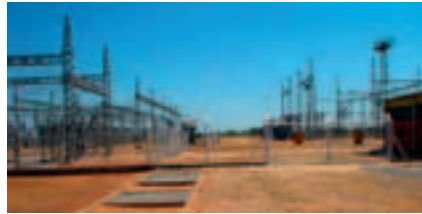
Gerus – high voltage direct current substation, Namibia
