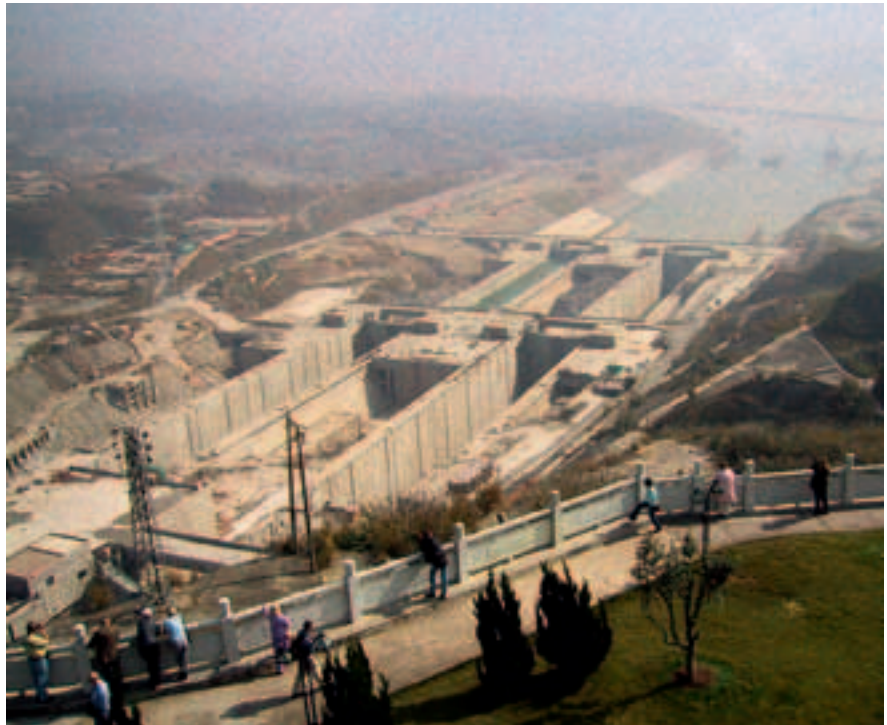
Image 1: The ship lock system of the Three Gorge Dam during construction (November 2002).
