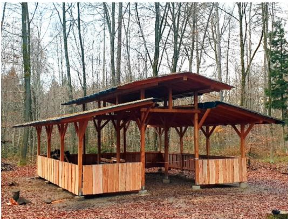
FIGURE 3 | Measurable delivery of the project Forest Classroom : The building under construction and completed.
