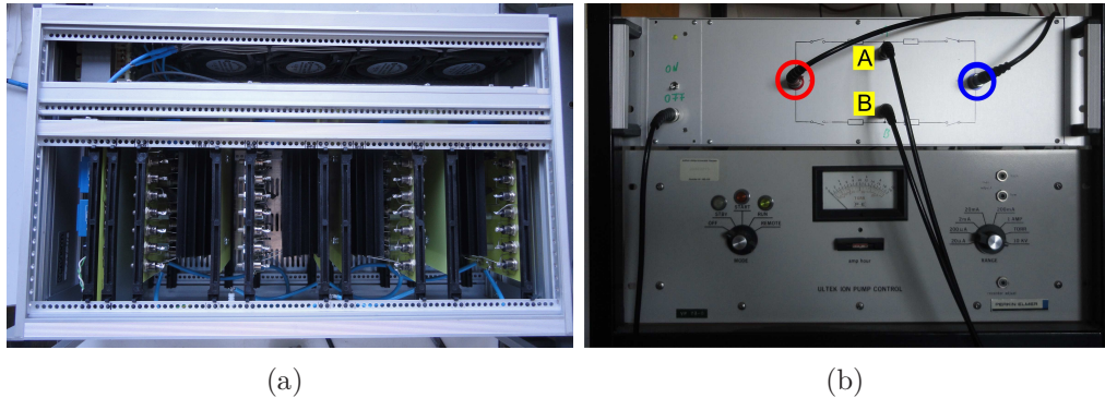
Figure 5.16: Figure a) shows a top view inside of the AC generator assembled by H. Weigand (Institute of Physical Chemistry). Figure b) shows in the upper part the front view of the AC generator with simple schematics of the cable connections: red and blue high voltage input, A and B connection to the electrodes of the dielectric plates and on the left bottom function generator input. Below the AC generator the high voltage source (power supply of a vacuum pump) can be seen.
